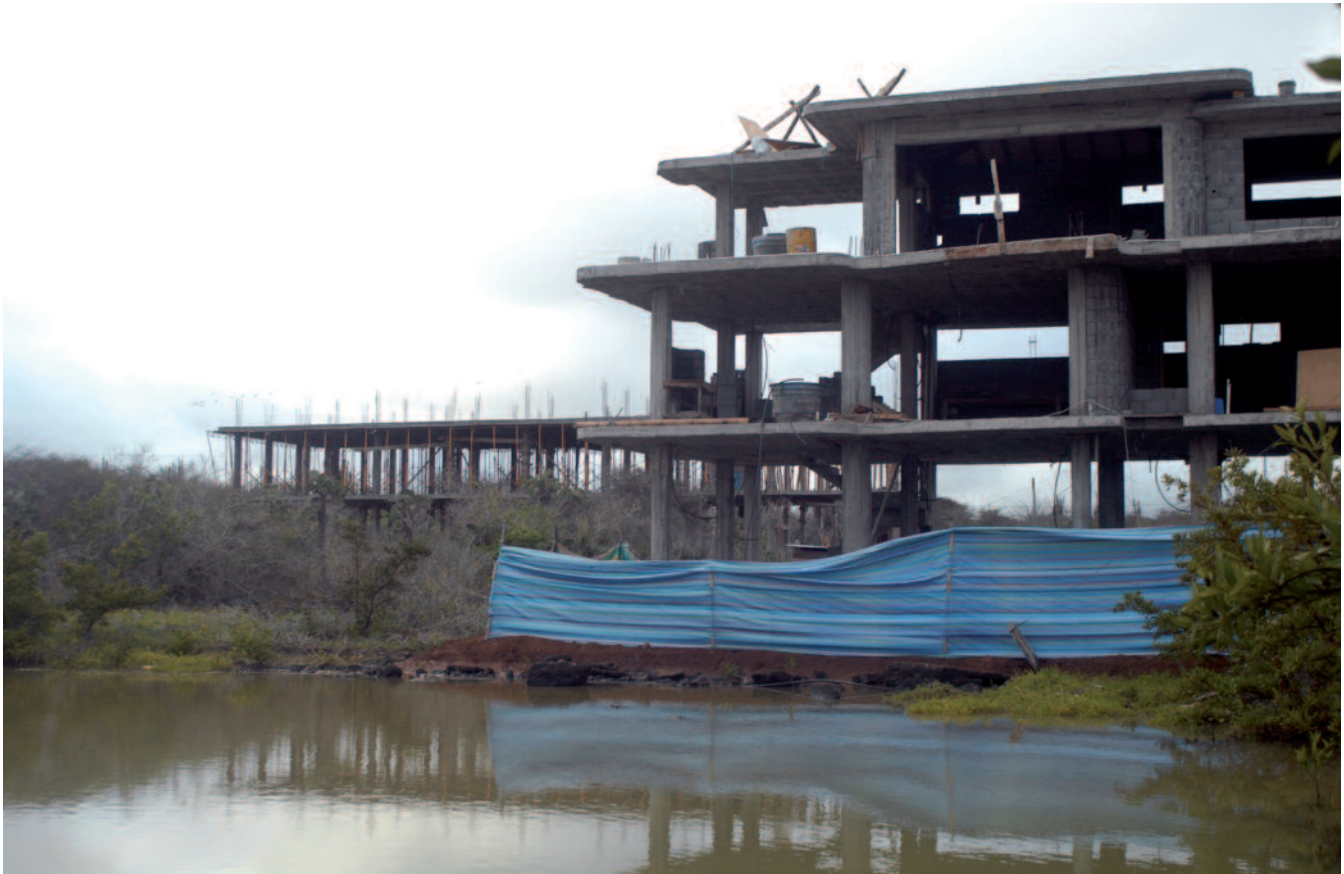
Photo 2. Destruction of the natural landscape in the last preserved neighborhood of Puerto Ayora, “Barrio Estrada”: construction of a house and a hotel. Photo: C. Grenier.
